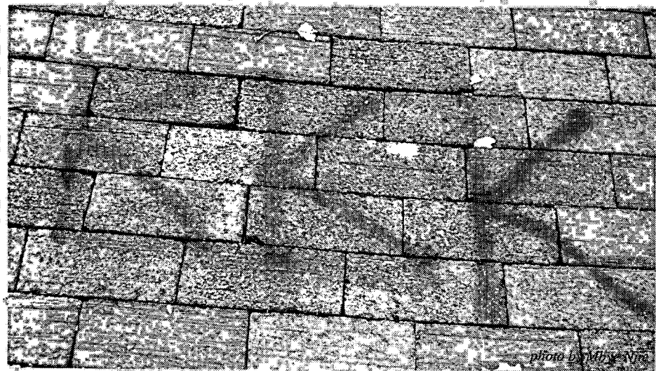
Vandals spray-painted the brick sidewalk in front of the laundry.
